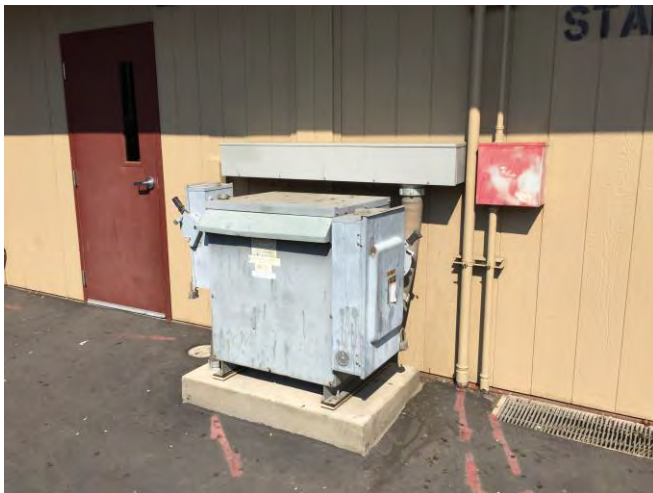
Photograph 13. (looking northeast). Small transformer on the western exterior wall of food service building.
