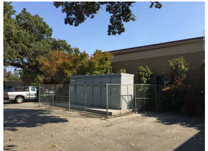
Photograph 14. (looking southeast). Electrical switch gear along northern exterior wall of library building.
