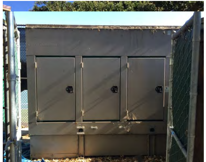
Photograph 6 (looking north). Emergency generator south of tennis court in Area 1.
